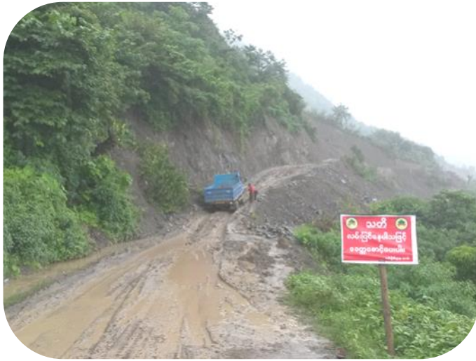
Road parts damaged by the landslides and surface water as a result of heavy rainfalls in Chin State. ©WFP/ Hien Adjemian.
